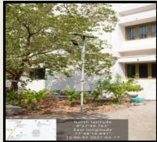
Solar Street Light – IT Block (West)
